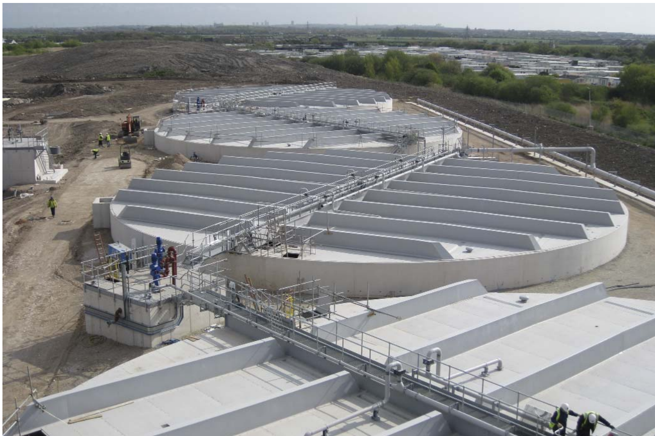
Primary settlement tanks and de-sludging chamber
