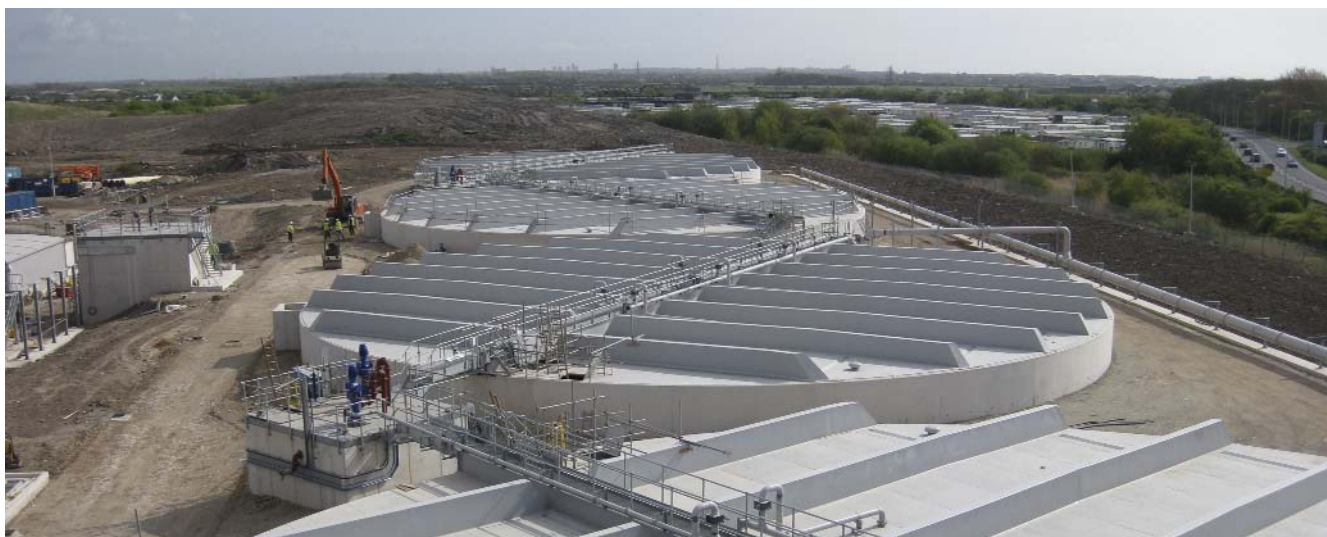
Primary settlement tanks and de-sludging chamber
