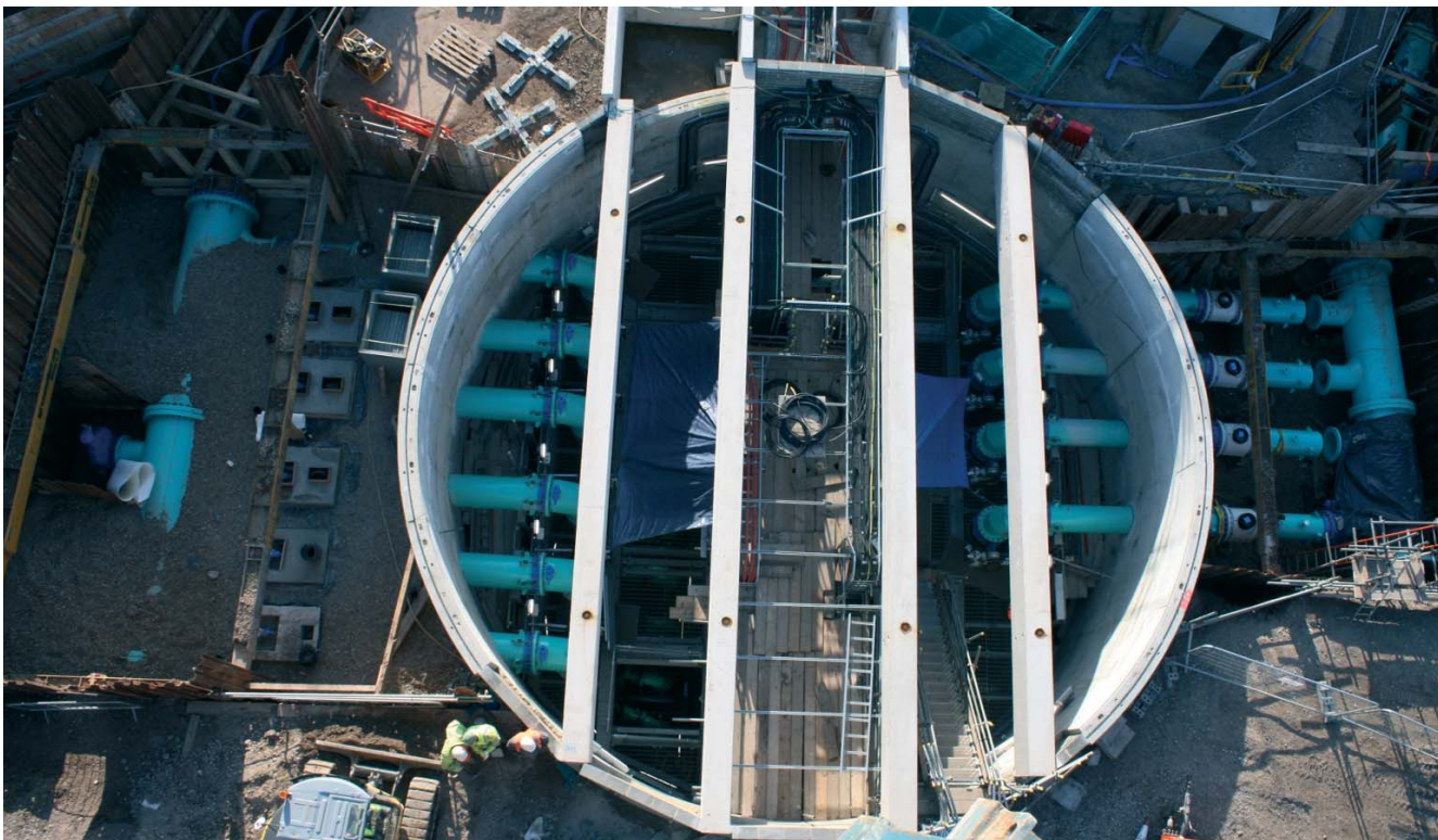
A high volume of existing buried services added to the challenge of pump-out shaft connections
