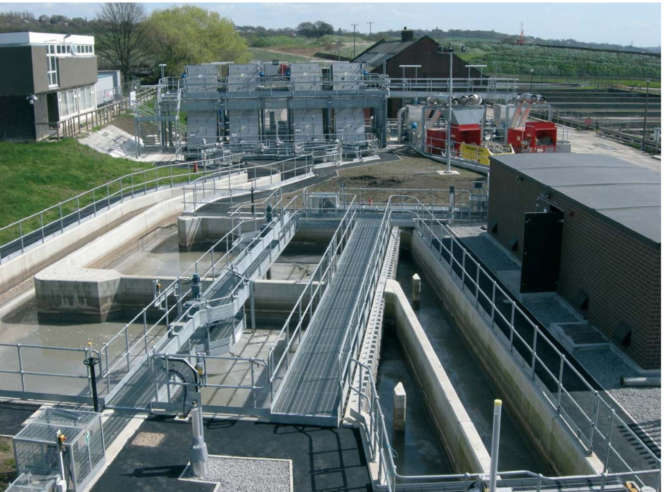
Mitchell Laithes WwTW Inlet Works
