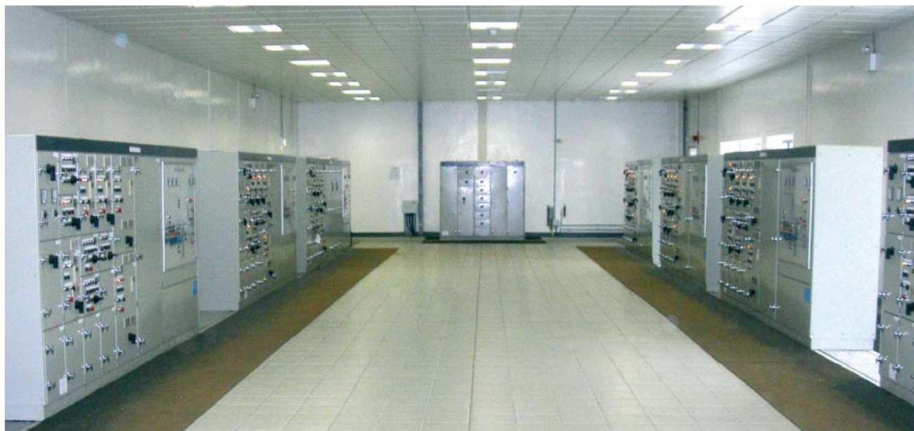
One of Carmoney's many switchrooms
