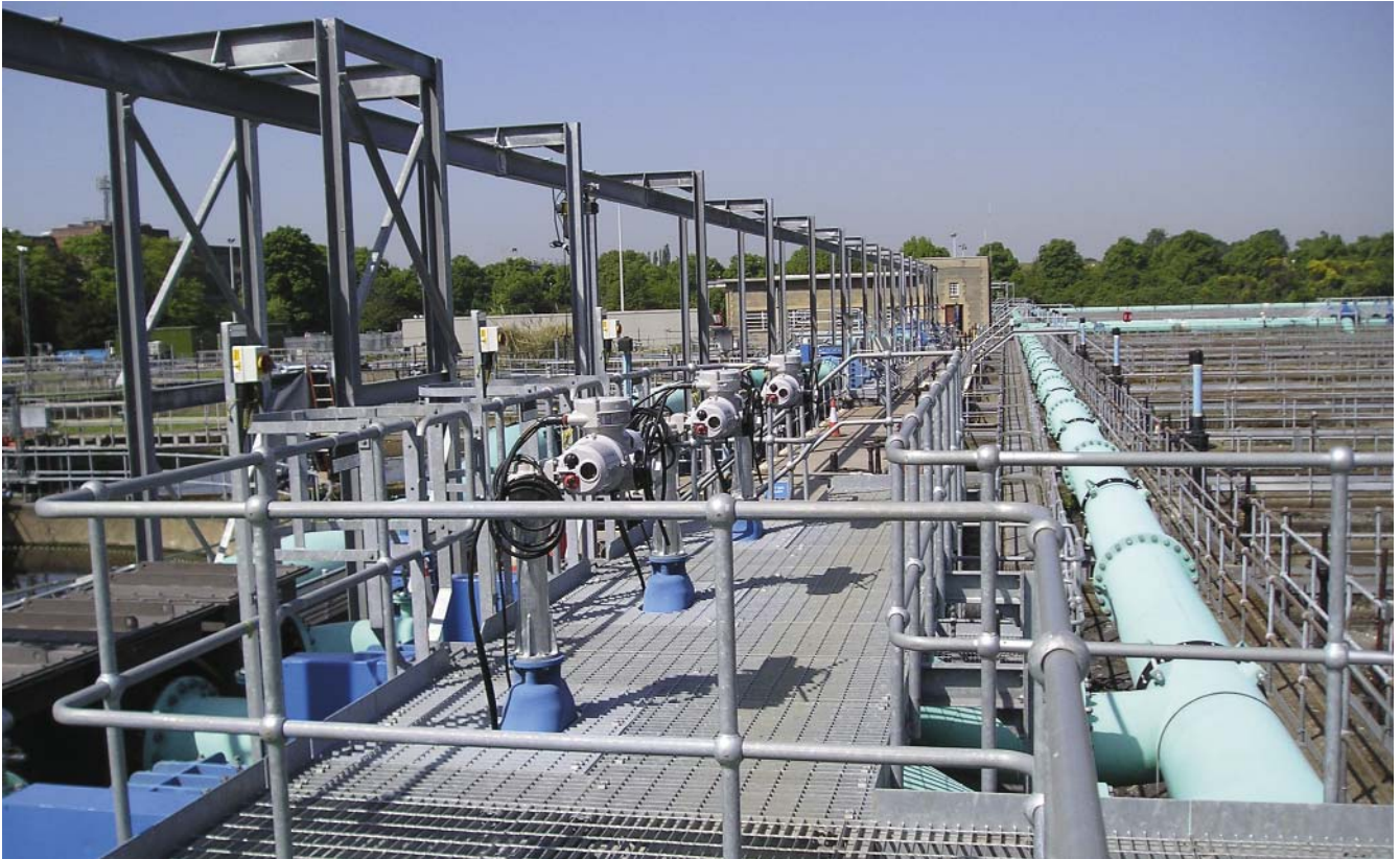
Maintenance Gantry for Mixed Liquor Pumping Stations
