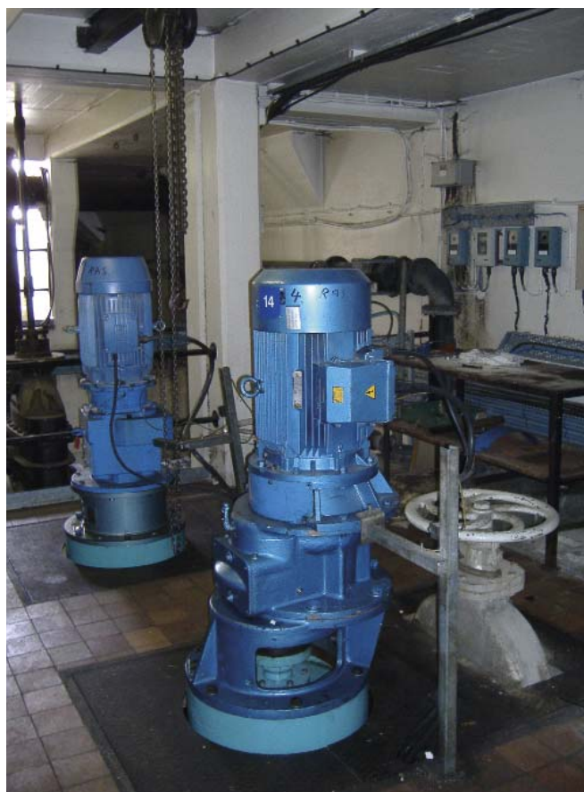
Mogden Battery C RAS Pumps Located within Subterranean Gallery Courtesy of Bewater Treatment Ltd
