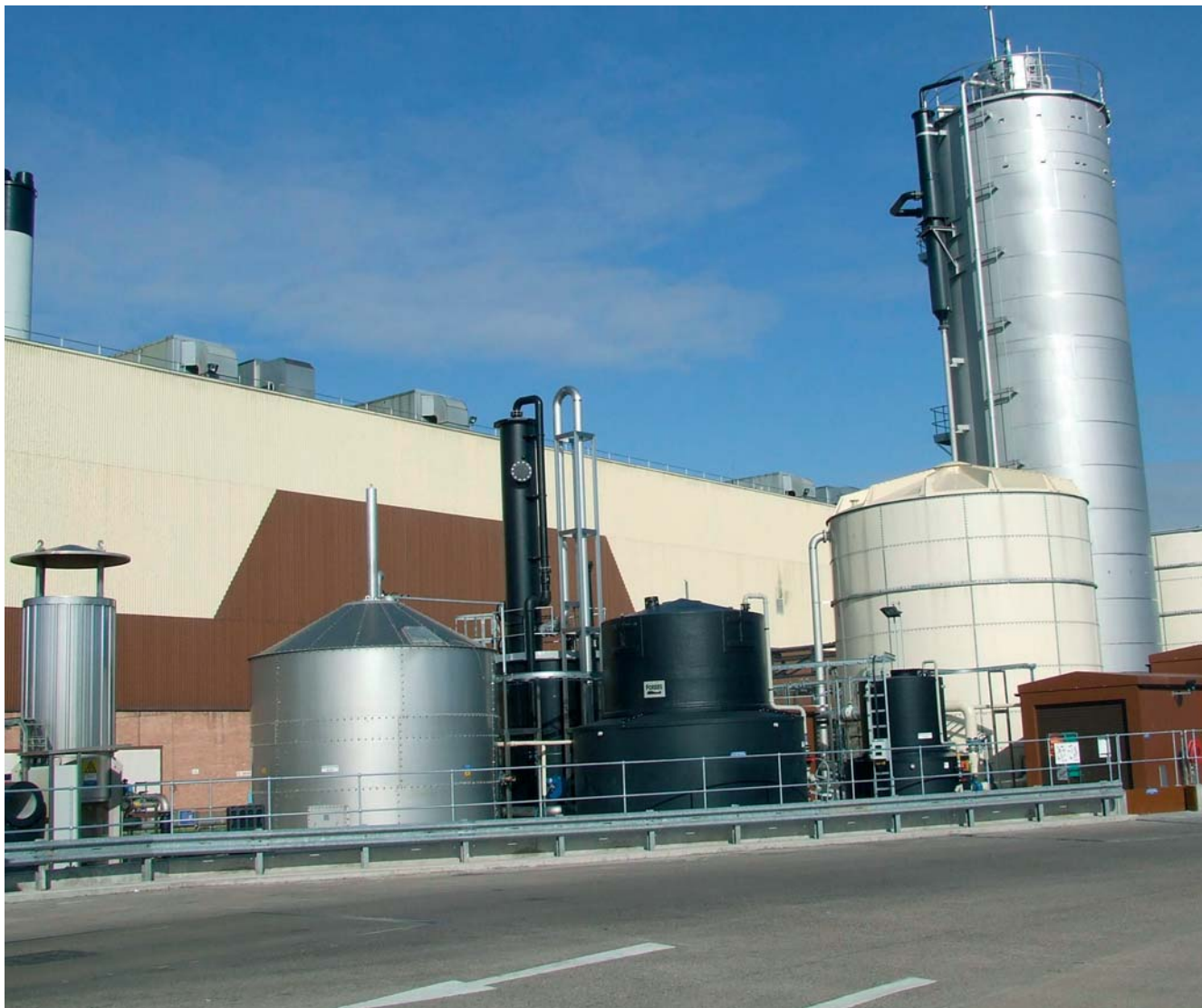
Anaerobic wastewater treatment plant
