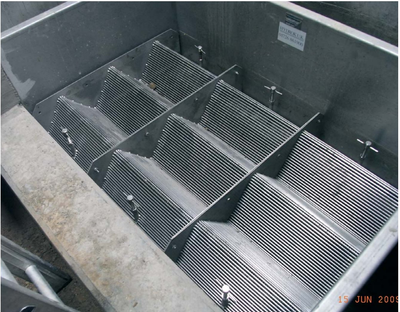
Static screen at West Holborn CSO located in South Shields
