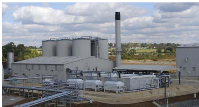
Great Billing – Monsal EEH plant, heating building, CHP's and waste heat boilers Courtesy of Galliford Try Meica JV Ltd
