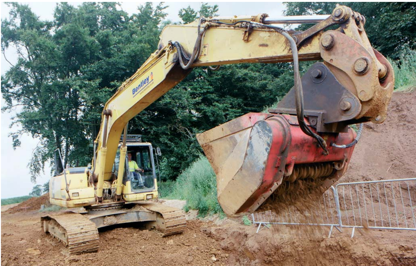
A processing bucket breaking up the soil being used to backfill around the pipe
