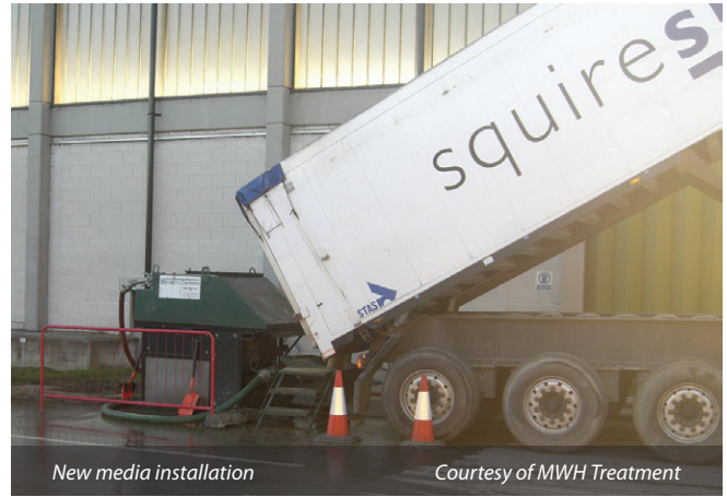
Washing the under floor laterals Courtesy of MWH Treatment
