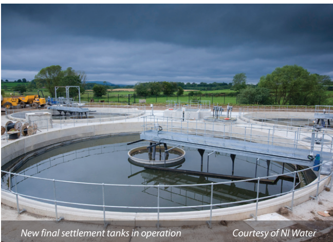
Site finishing around the intermediate settlement tanks and odour control slab - Courtesy of NI Water
