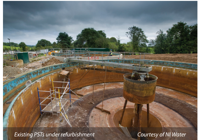
Existing secondary filters prior to refurbishment Courtesy of NI Water
