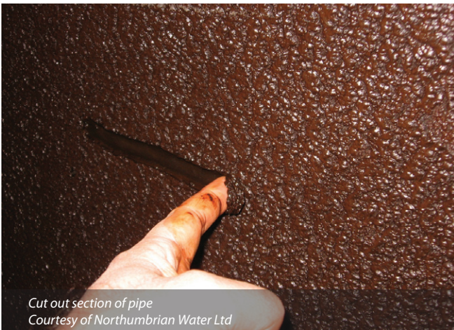
Under pressure coupon Courtesy of Northumbrian Water Ltd
