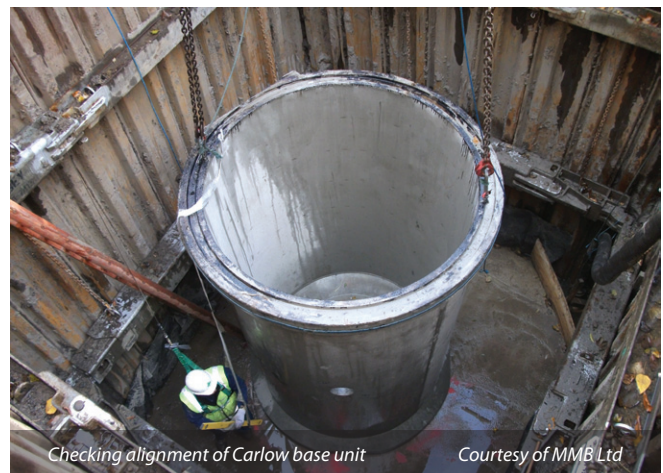
Carlow base unit being lowered into excavation at Bolton on Swale Courtesy of Mott MacDonald Bentley Ltd
