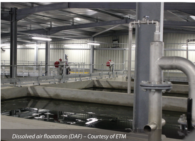
Dissolved air flotation (DAF) plant area – Courtesy of ETM
