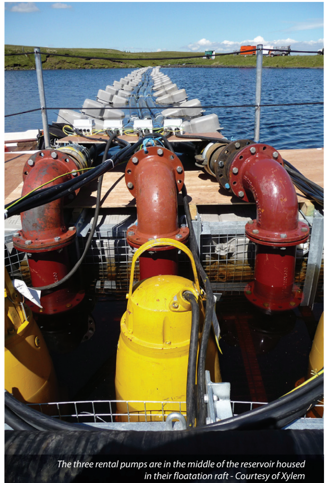
The key logistical issue was how to get the equipment to the reservoir up a dirt track in terrible weather conditions - Courtesy of Xylem
