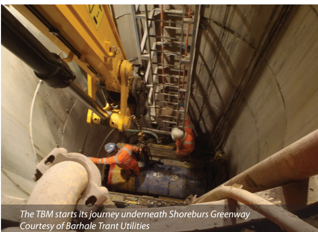
The TBM is lowered into the shaft Courtesy of Barhale Trant Utilities
