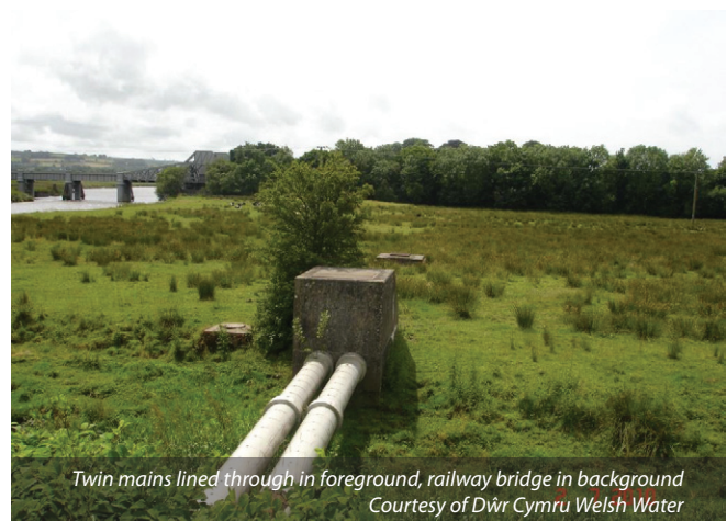
River Towy next to Pothouse Wharf SPS Courtesy of Dŵr Cymru Welsh Water
