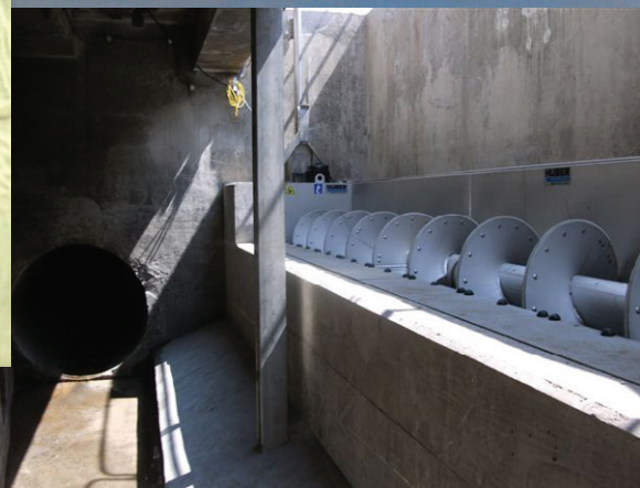
New screen at Pothouse Wharf Courtesy of Dŵr Cymru Welsh Water
