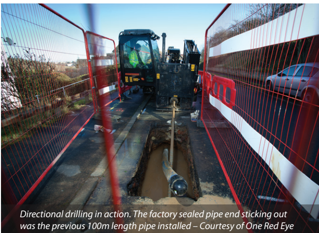
Barriered off service transfer excavations in road. Note existing services marked up on the footpath with spray paint – Courtesy of One Red Eye
