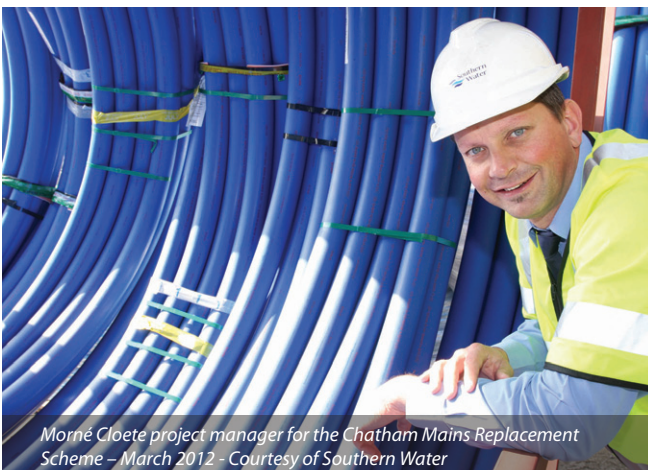
MDPE pipe being pulled through behind the reamer attached to the directional drilling head – Courtesy of One Red Eye
