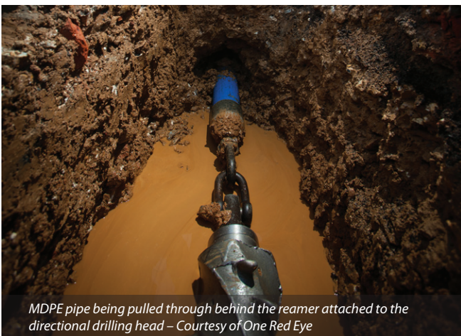
Directional drilling in action. The factory sealed pipe end sticking out was the previous 100m length pipe installed – Courtesy of One Red Eye
