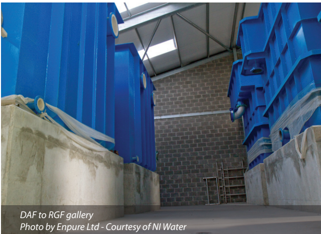
DAF and Flocculation tanks prior to cladding Photo by Enpure Ltd - Courtesy of NI Water
