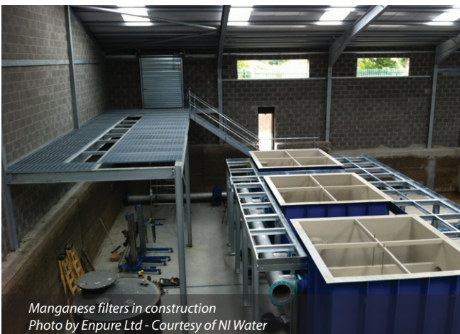
DAF to RGF gallery Photo by Enpure Ltd - Courtesy of NI Water
