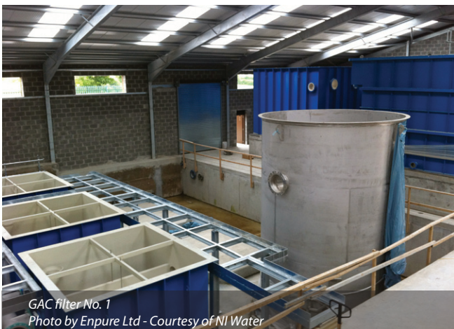
Manganese filters in construction Photo by Enpure Ltd - Courtesy of NI Water
