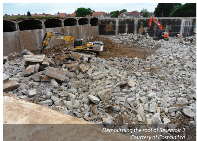
Crushing the concrete arising from the Reservoir 3 roof slab with a Dust Boss dust suppression system in place - Courtesy of Costain Ltd
