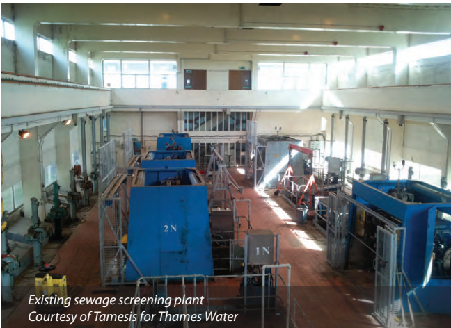
Existing sewage pump transfer system Courtesy of Tamesis for Thames Water
