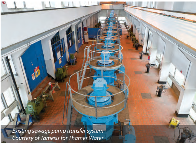
Existing works adjacent to the Thames and SPG Courtesy of Tamesis for Thames Water
