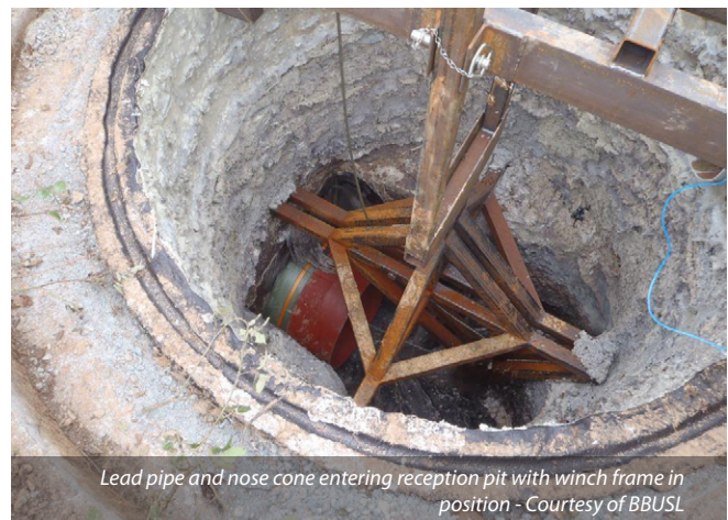
Excavated collapse section. The wall thickness had eroded to 12mm Courtesy of BBUSL
