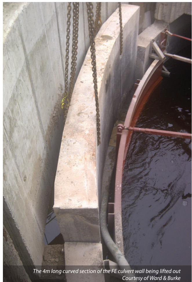
The culvert roof removed with the flume in place Courtesy of Ward & Burke
