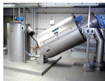
Drum Thickeners and Dewaterers
