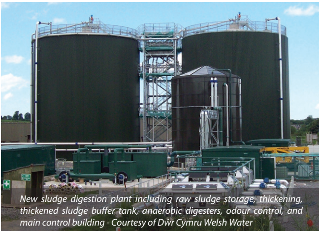
Five Fords Anaerobic Digestion plant including membrane gas holder and high efficiency CHP units - Courtesy of Dŵr Cymru Welsh Water
