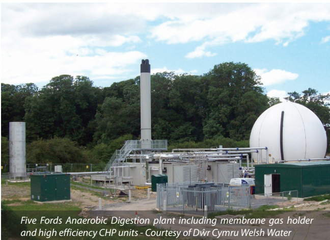
Complete sludge digestion plant Courtesy of Dŵr Cymru Welsh Water
