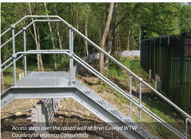
Plastic sheet piles installed in the existing flood embankment at Bryn Cowlyd WTW - Courtesy of Waterco Consultants
