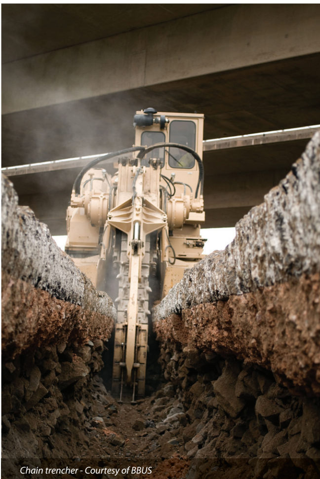
Ground guard system used to protect Newport Park, an environmentally sensitive area - Courtesy of BBUS
