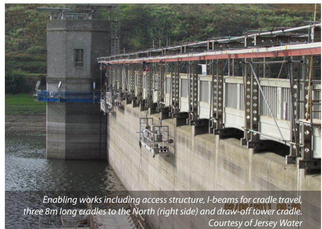
The south (left) abutment partially completed. Sacrificial textile and drainage geonet is in place - Courtesy of Jersey Water
