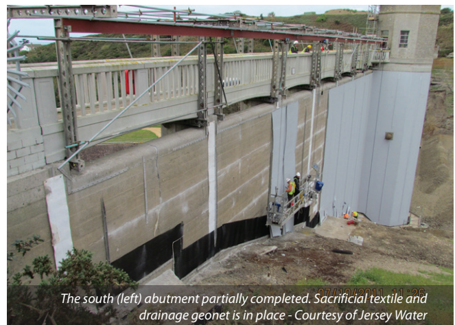
Hanging the geomembrane on the draw-off tower. The membrane is lifted upwards from the base of the tower. Note sacrificial textile is placed on the corners of the tower to protect the geomembrane. Courtesy of Jersey Water
