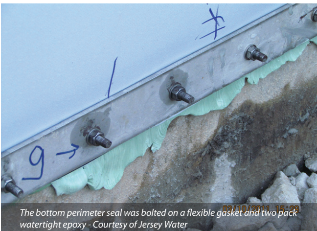
This view shows the open channel section of the tensioning profile (centre). The lower 1m of is fitted with a black geonet to enhance drainage. The bottom perimeter seal is temporarily fixed for drilling the anchors - Courtesy of Jersey Water
