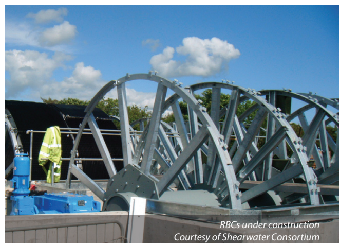
Keady WwTW - Phase 2 complete - January 2012 Courtesy of Shearwater Consortium
