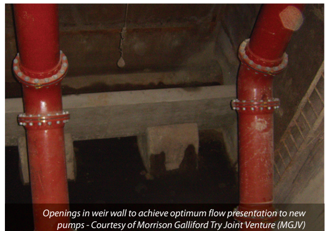
New pump access openings/covers Courtesy of Morrison Galliford Try Joint Venture (MGJV)
