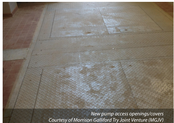
Original layout of assets. DWF pump motors located on far end of room. Original MCC (immediate left) located opposite the storm pumps Courtesy of Morrison Galliford Try Joint Venture (MGJV)
