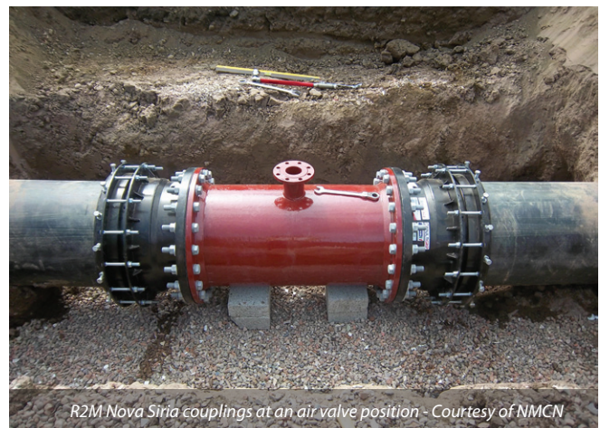
Pipe bridge - Courtesy of NMCNomenca
