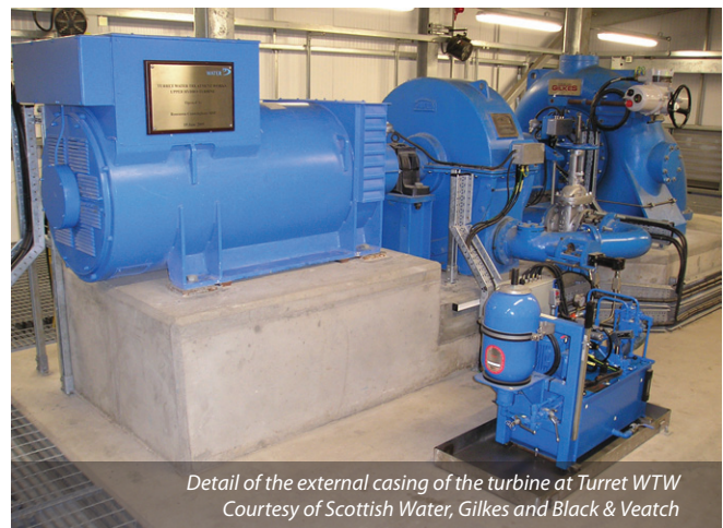
A Gilkes turbine installed at a WTW by Black & Veatch Courtesy of Scottish Water, Gilkes and Black & Veatch
