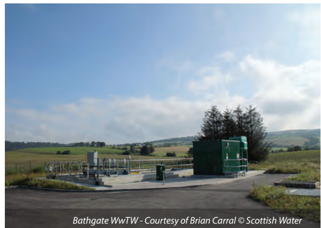
Linlithgow WwTW - Courtesy of Brian Carral © Scottish Water
