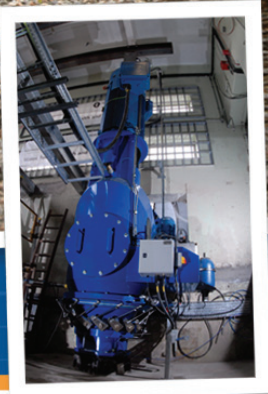
Mosswood WTW Hydro Turbine, County Durham
