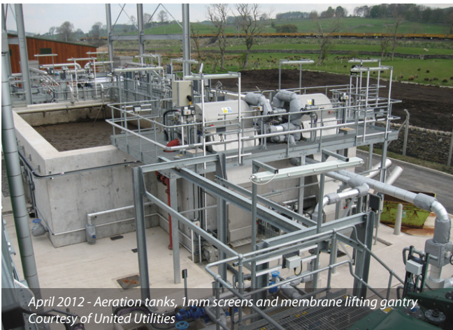
Reversible permeate pumps in main plant building Courtesy of United Utilities
