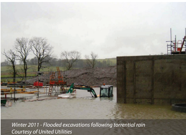
Shap WwTW July 2011 - Courtesy of United Utilities
