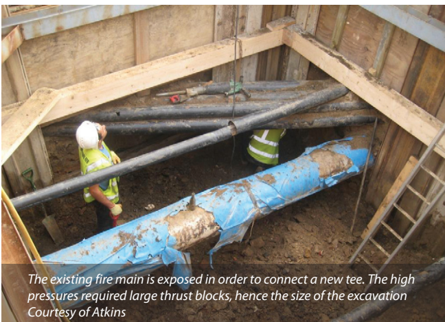
Atkins brought in specialist testing equipment to undertake an assessment of the existing network's serviceability. - Courtesy of Atkins
