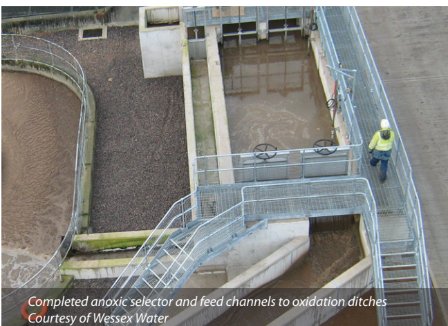
New oxidation ditch operating alongside existing ditch Courtesy of Wessex Water
