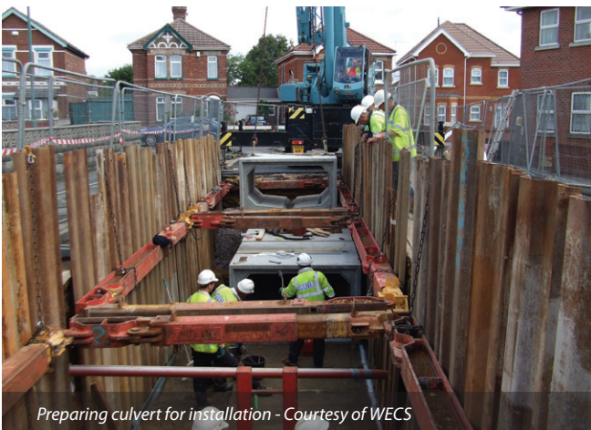
Culverts and rider sewer - Courtesy of WECS
