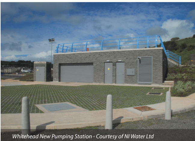
Whitehead New Pumping Station (from viewing platform facing north) Courtesy of NI Water Ltd
