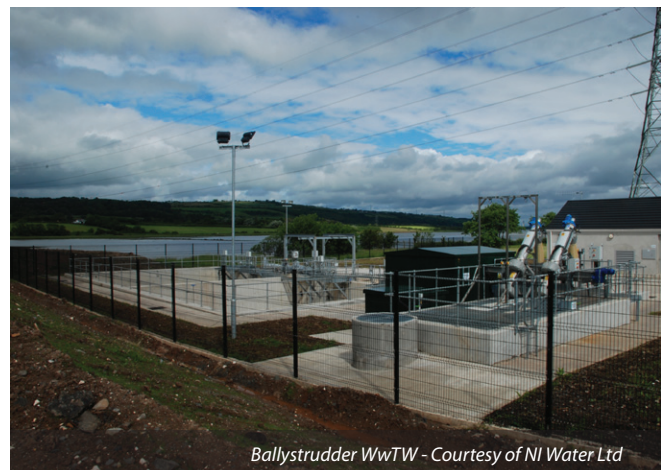
Ballycarry WwTW - Courtesy of NI Water Ltd
