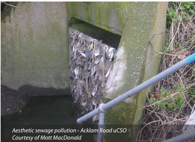
Aesthetic sewage pollution - Old River Tees watercourse Courtesy of Mott MacDonald
