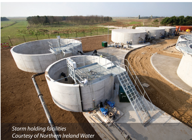
View from upstream of PSTs and flow split chamber Courtesy of Northern Ireland Water
