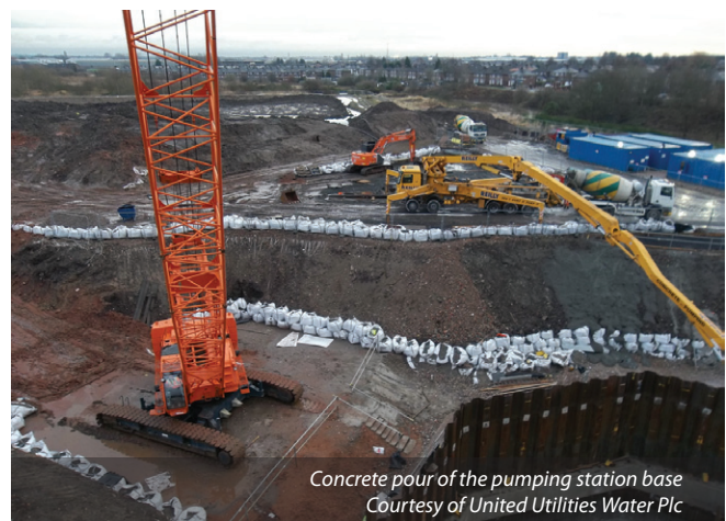
Shaft excavation showing the hydraulic shores installation (Intermediate beam level) - Courtesy of DCT Civil Engineering Ltd
