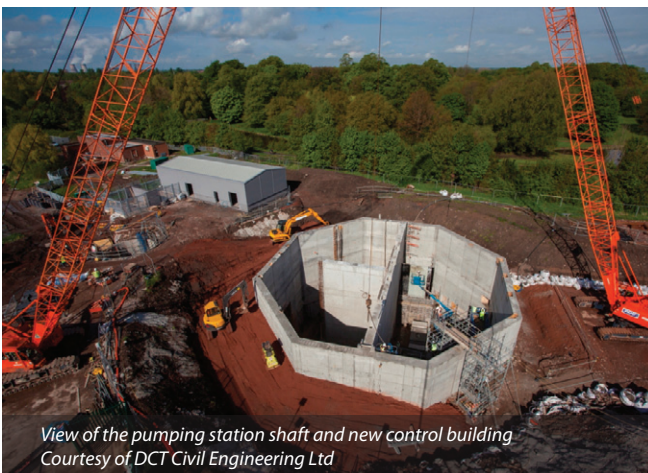
New control building & pumping station inlet manhole and the existing pumping station building - Courtesy of DCT Civil Engineering Ltd
