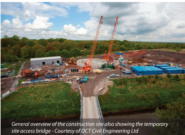
View of the pumping station shaft and new control building Courtesy of DCT Civil Engineering Ltd
