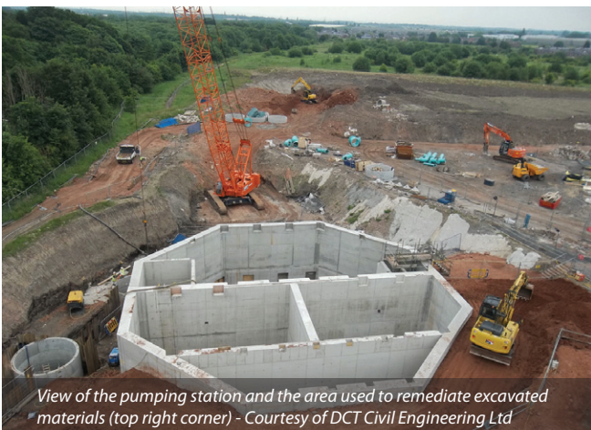
General overview of the construction site also showing the temporary site access bridge - Courtesy of DCT Civil Engineering Ltd
