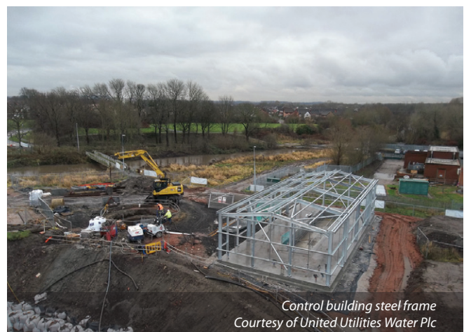
Concrete pour of the pumping station base showing intermediate concrete beam and part of the wells internal walls steelworks Courtesy of United Utilities Water Plc
