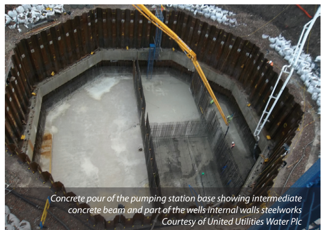
Concrete pour of the pumping station base Courtesy of United Utilities Water Plc
