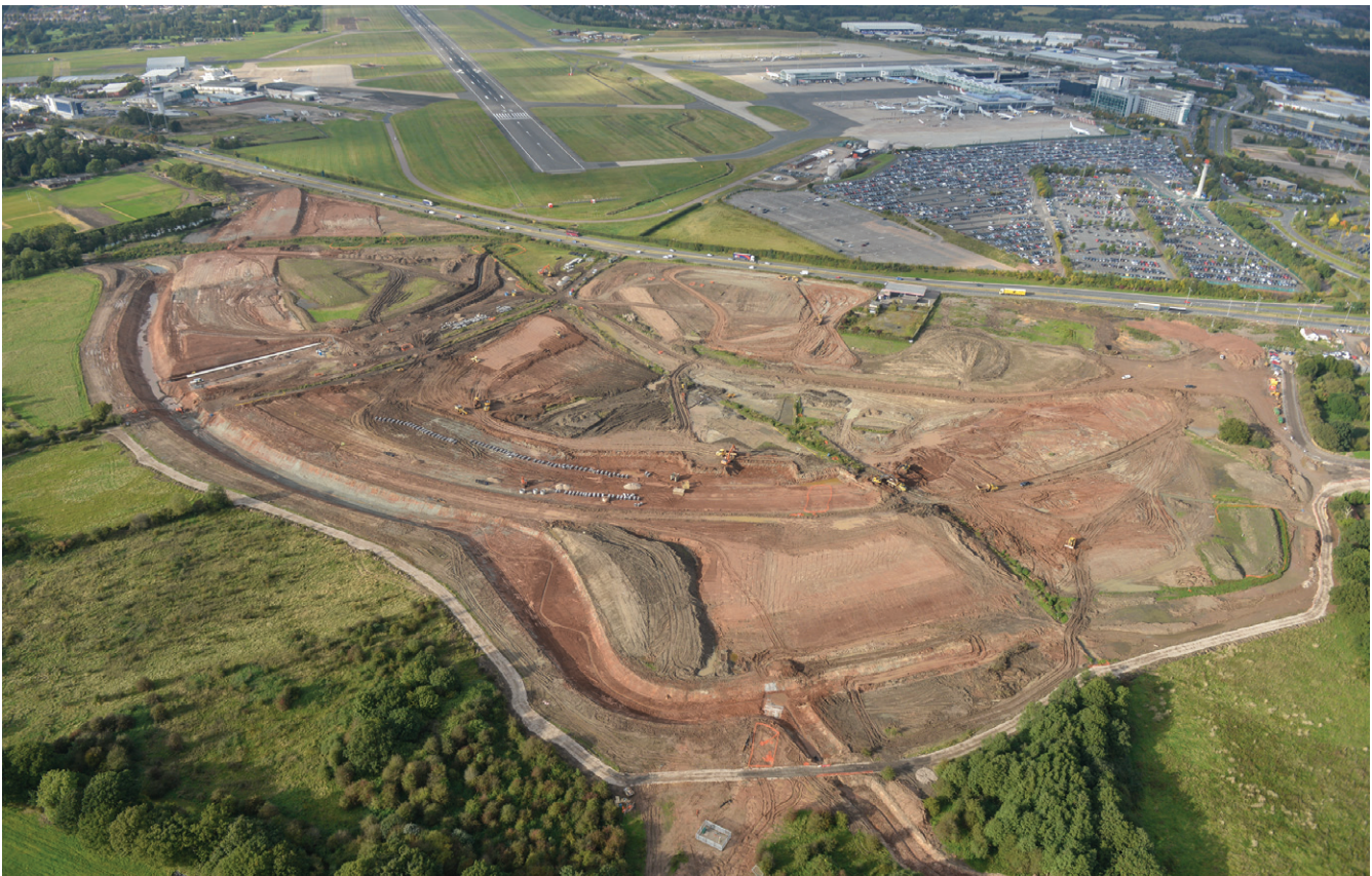
Aerial photograph of the site, early in the works programme - Courtesy of Volker Fitzpatrick Colas
