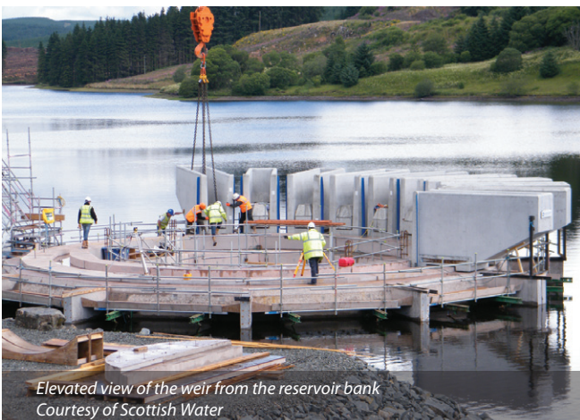
The pontoon and valve tower, with the spillway to the right Courtesy of Scottish Water
