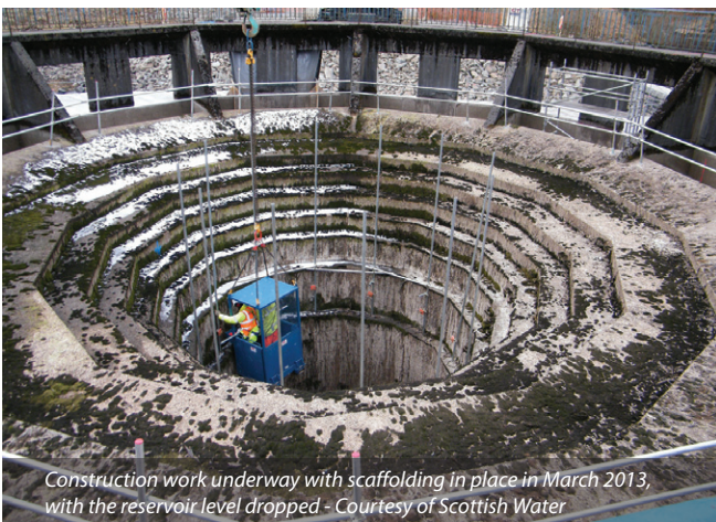
The spillway prior to construction of the new circular piano-key weir Courtesy of Scottish Water
