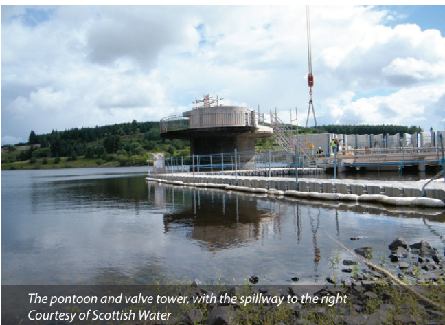
Construction work underway with scaffolding in place in March 2013, with the reservoir level dropped - Courtesy of Scottish Water
