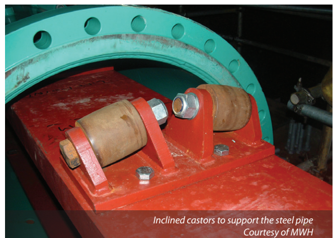
The fifth steel pipe is carefully inserted into the tunnel Courtesy of MWH
