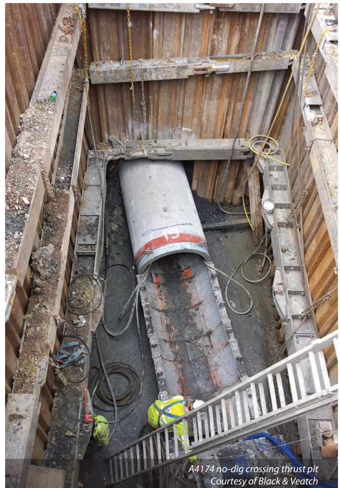
Long crossing of a 9" cast Iron distribution main feeding 150,000 customers - Courtesy of May Gurney
