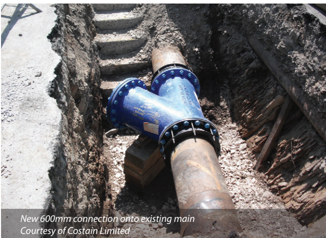
Valve thrust chamber pipework and steel reinforcements Courtesy of Costain Limited
