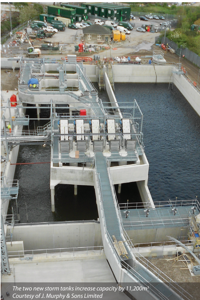
The detritors and inlet works remove rag and grit Courtesy of J. Murphy & Sons Limited
