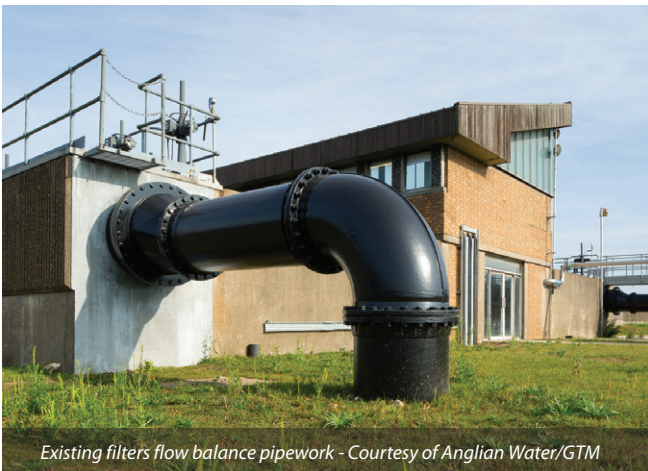
High rate lamella clarifiers - Courtesy of Anglian Water/GTM
