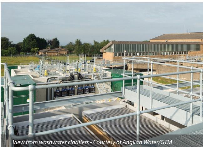
New rapid gravity filters - Courtesy of Anglian Water/GTM
