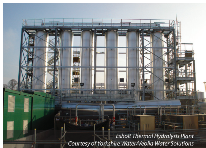
Existing AMP4 engine installation. New gas holder & waste gas burner in background - Courtesy of Yorkshire Water
