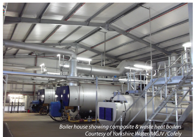
Esholt Thermal Hydrolysis Plant Courtesy of Yorkshire Water/Veolia Water Solutions
