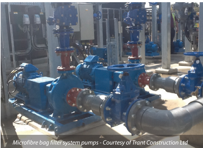
GAC filters and local supply and marshalling panels Courtesy of Trant Construction Ltd
