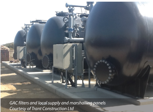
GAC filters and local supply and marshalling panels Courtesy of Trant Construction Ltd
