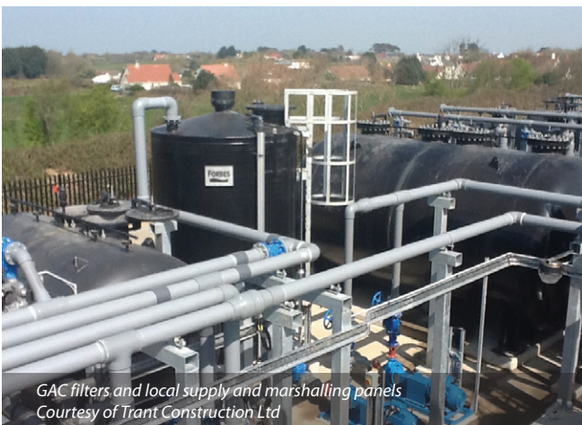
GAC filters & central pipework runs - Courtesy of Trant Construction Ltd
